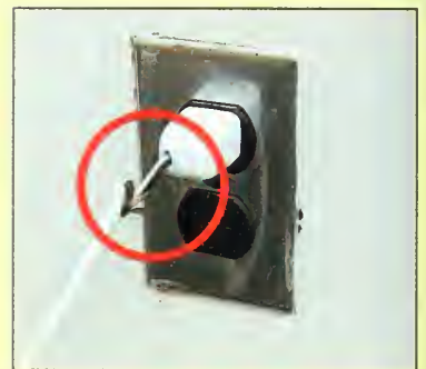
Inspectors found this frayed wire on a floor fan plugged into the wall of Mary's third-floor office. Check all the wires in your home; if any are damaged, they must be replaced.
